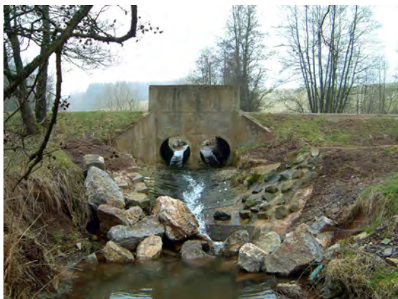
Figure 4a: A channelized crossing with unfavourable conditions for animals to migrate before reconstruction
